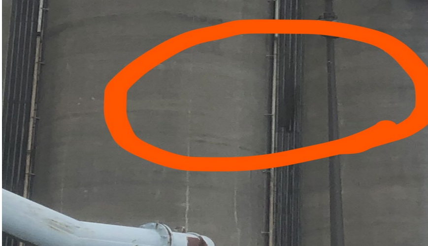
Figure 3: Silo 6 loose cladding
