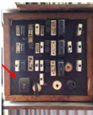
(Asbestos Containing Electrical Backing Board Example)
