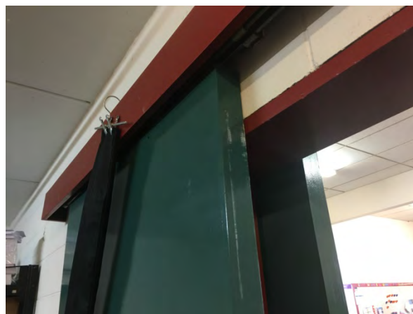
(Asbestos Containing Fire Door, Public Library Example)
