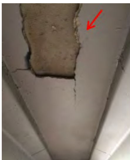
(Asbestos Containing Millboard Example)
