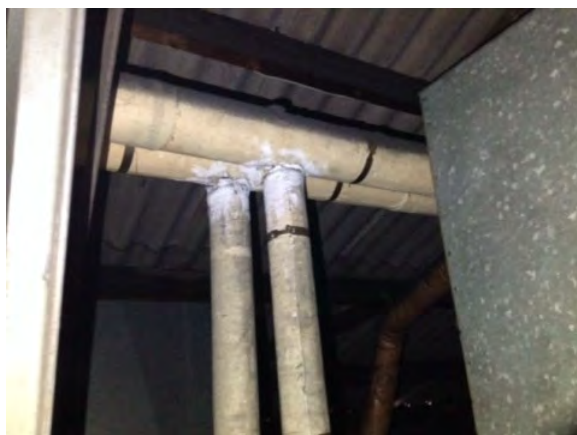
(Asbestos Containing Lagging Example)
