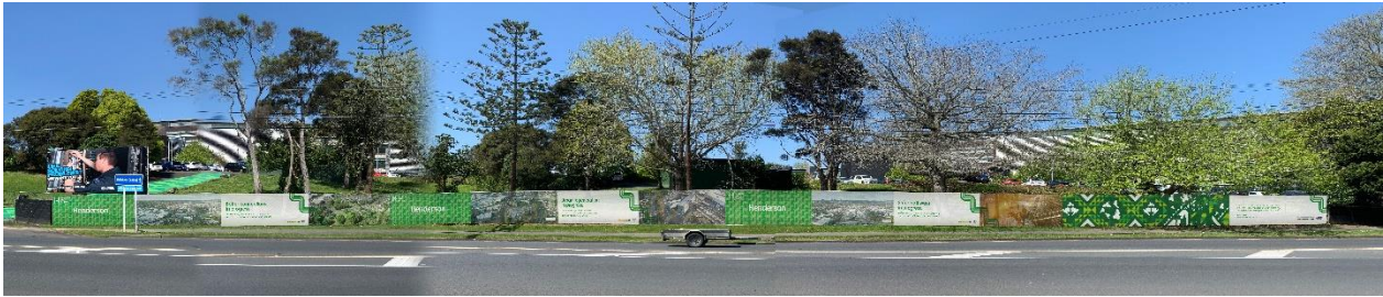
Figure 6: Subdivision works underway – Hoardings are up, showcasing the new local identity branding approach.
